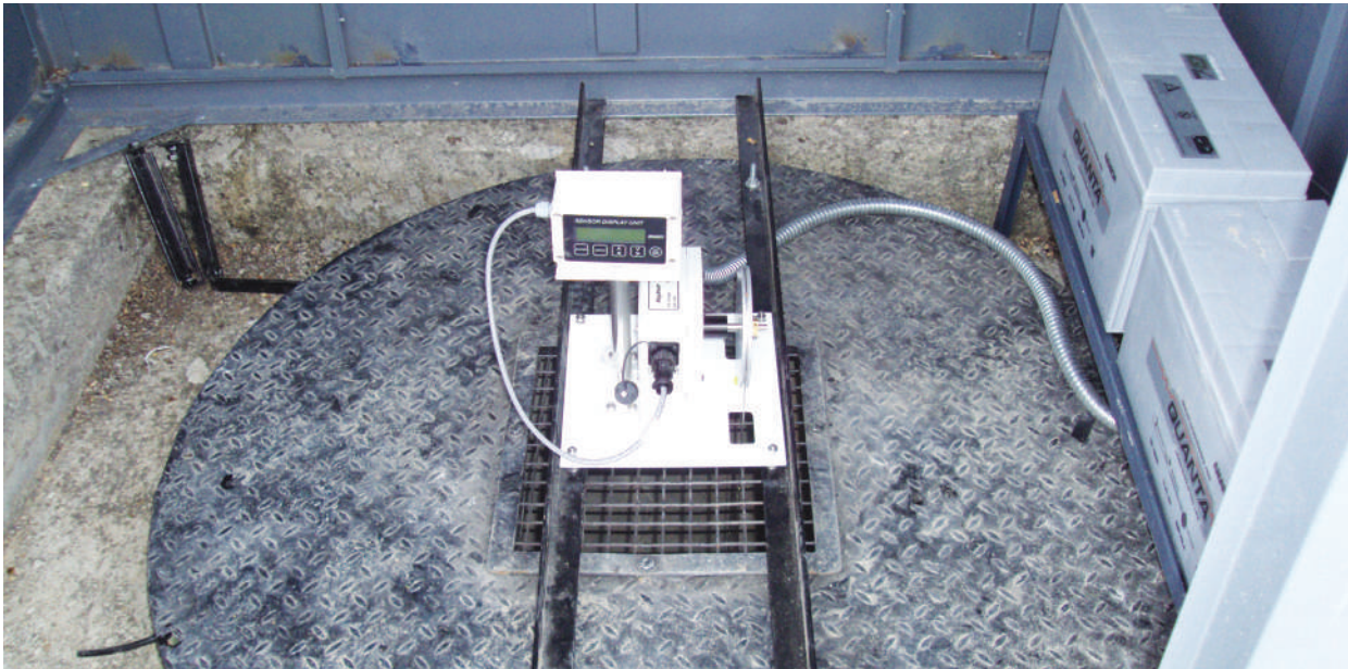
Figure 3.7: An example of a shaft encoder installed in Maharashtra
