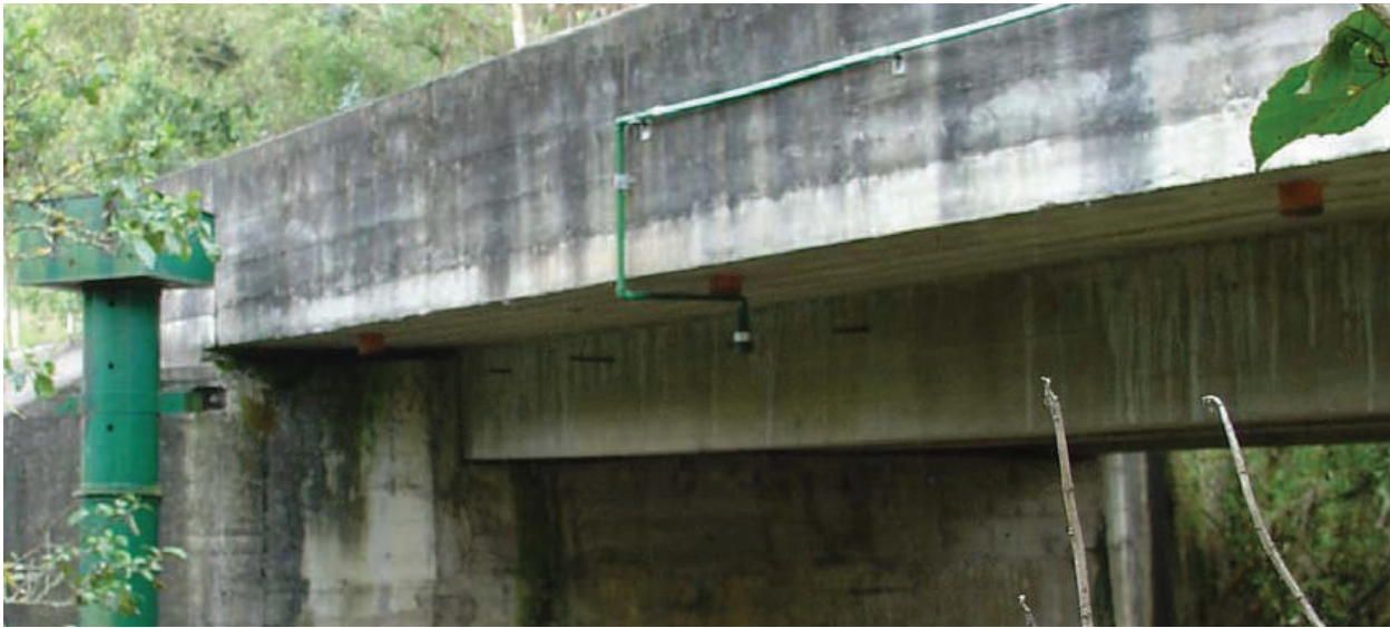
Figure 3.3: An ultrasonic sensor being used to measure water elevation using a bridge mount
