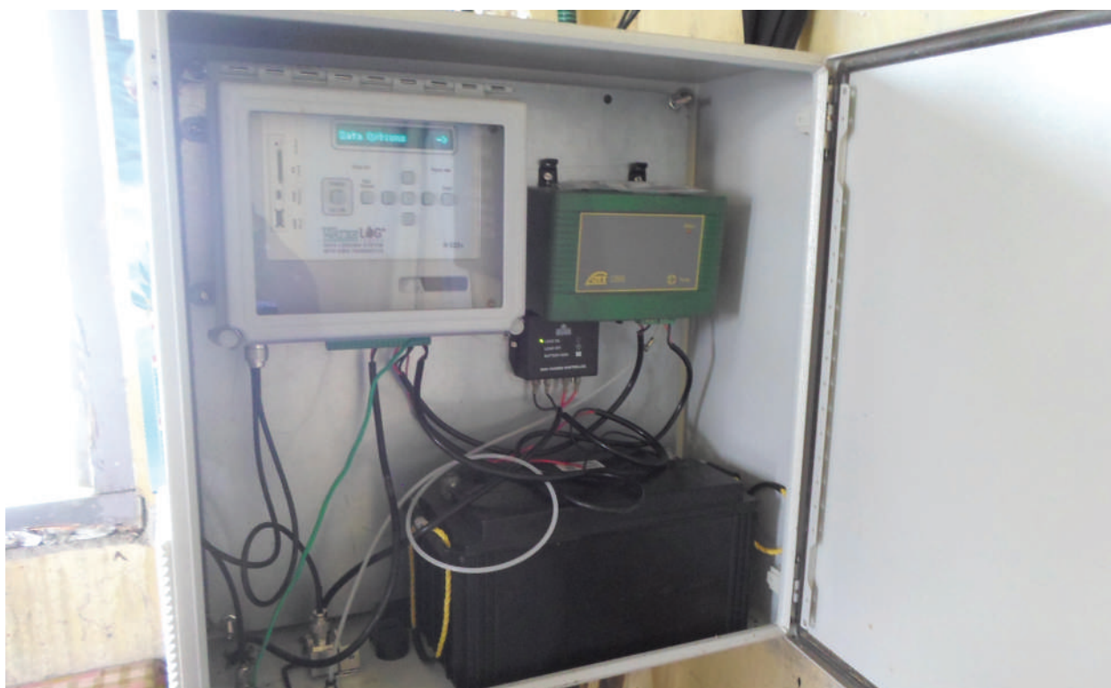
Figure 3.10: A bubbler system installed by CWC in Guwahati, Assam
