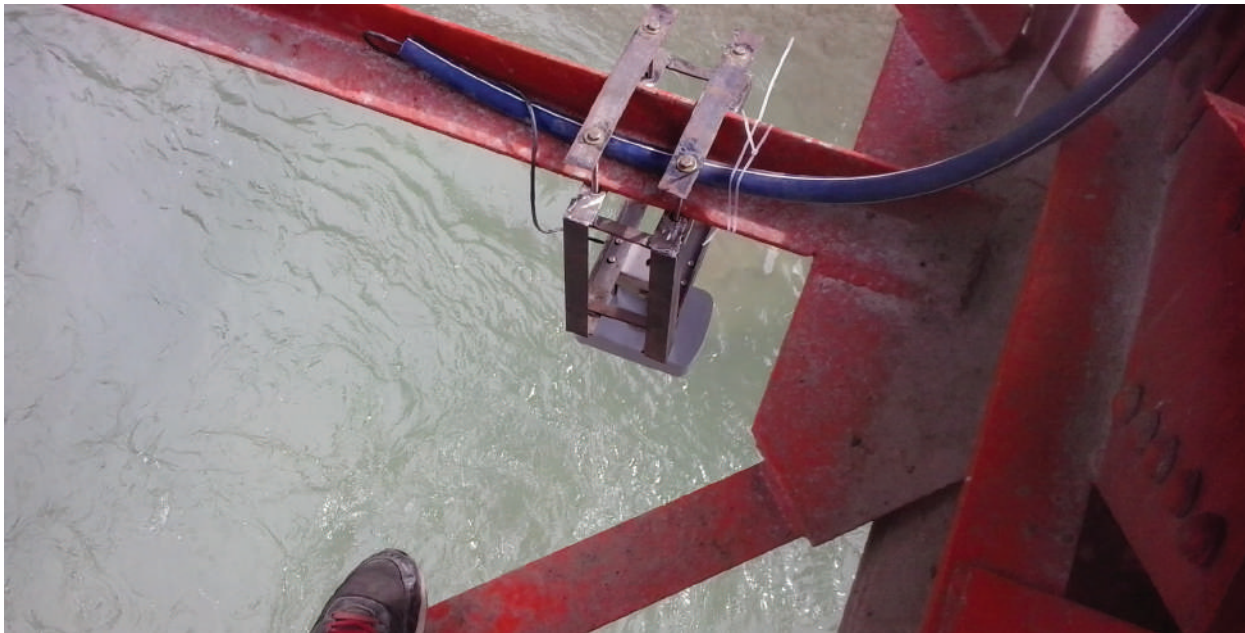
Figure 3.5: Radar sensor installed on bridge at Sainj in Himachal Pradesh by Bhakra Beas Management Board
